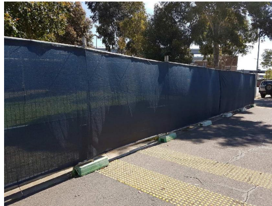
Figure 5 - Temporary fencing with shade cloth as a dust barrier (Refer AS4687:2007 Temporary Fencing and Hoardings)
