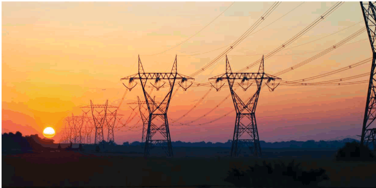
Figure 8: Power pylons in southeast Australia – climate change is worsening extreme weather including heatwaves and is placing ageing energy infrastructure under increasing stress.
