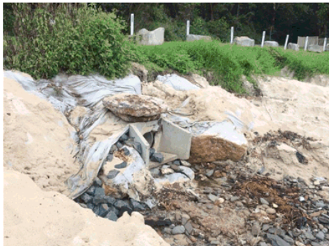
Photo 4: Central storm water outlet to be treated as part of the storm water upgrade
